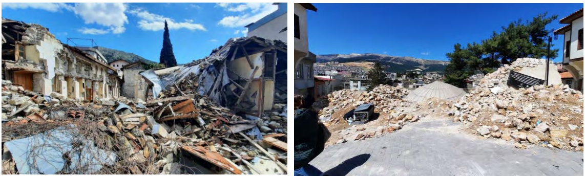
Fig. 5. Historical buildings in Hatay and Kahramanmaraş that collapsed and were heavily damaged after the earthquake [16]
